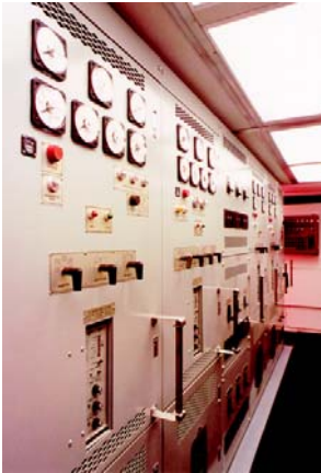
SCR机房内视
